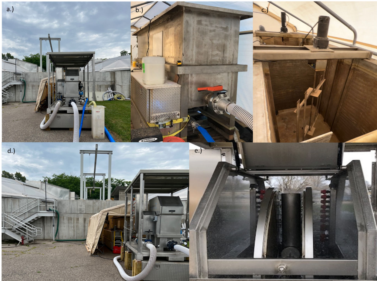
Figure 3. Pilot Setup: a.) Pilot Unit with Clarifier in the background, b.) Two-Stage Flocculation Tankage, c.) Internal View of Flocculation Tank, d.) Ultrascreen Pilot Overall, e.) View of Ultrascreen Disks and Backwash System
